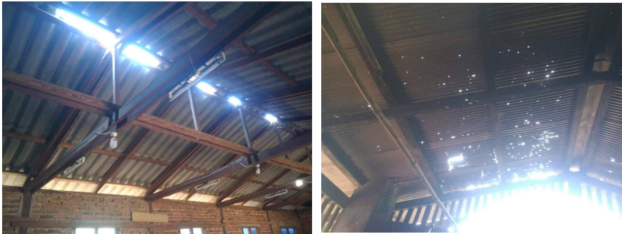
Leaking tin roof and the storm tored roof.
